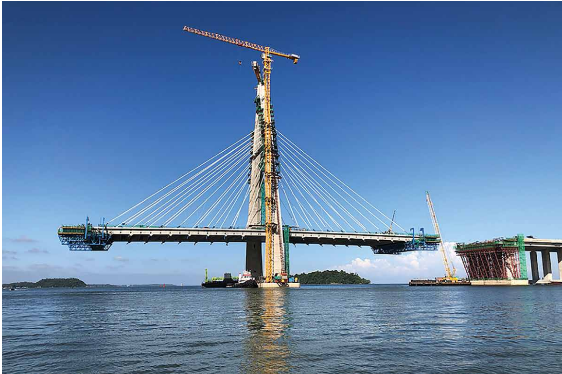
Part of China’s Belt and Road Initiative, the partially completed bridge at the Kota Batu end of the Temburong Bridge construction project in Brunei. (Peter L. Higgs)
