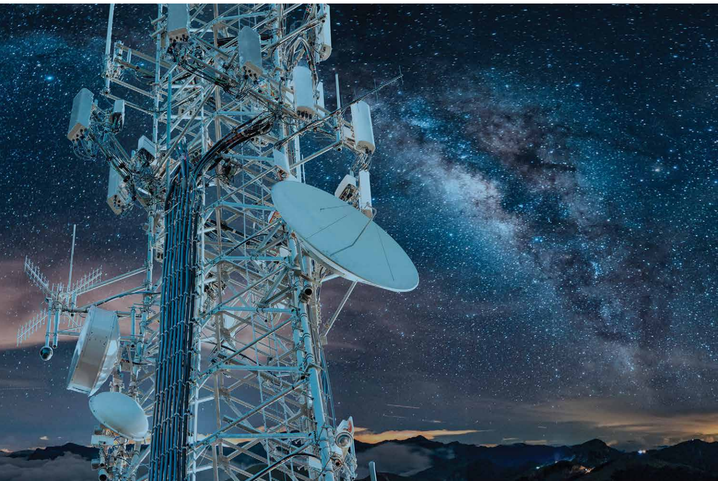
5G Repeater Tower, Mobile Phone Base Station. (Bill Oxford)
