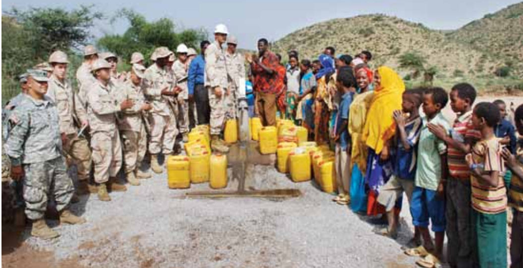
Naval Mobile Construction Battalion and Army CA team members celebrate with locals on completion of new well
